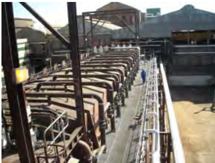
Lateral view with juice distributors feeding pipes
